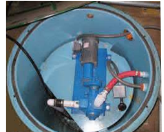
High-performance oil/water separator with influent pump packages
