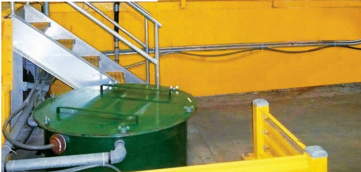
deep sump basin
